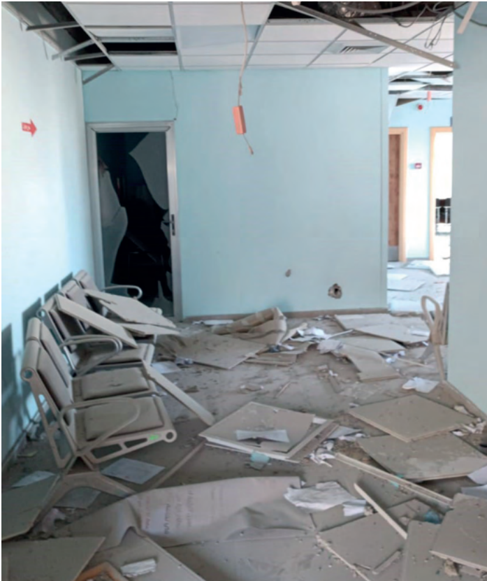
The interior showing collateral damage at SJEHG's Gaza Hospital
